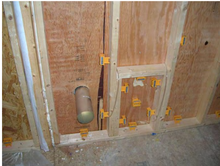
Wireless moisture sensors installed in the plywood stud bay with the dryer vent
