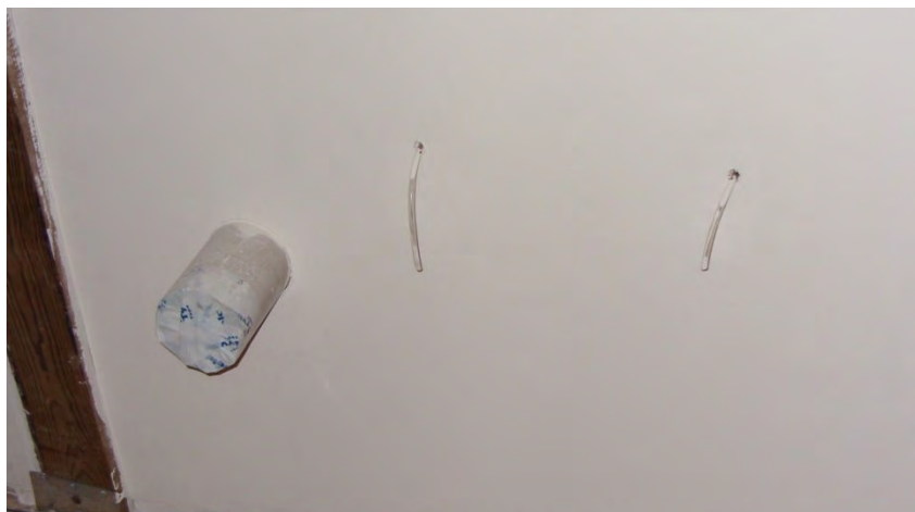
Figure 2: Interior face of one wall showing dosing tubes, and dryer vent penetration
