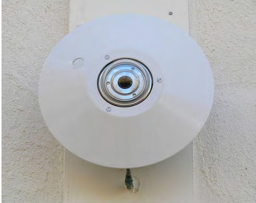
Vertical pyrometer located on wall surface
