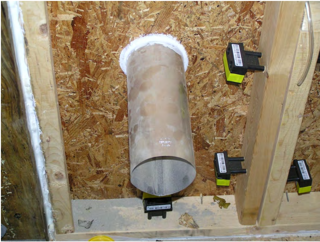
Wireless moisture sensors installed in an OSB stud bay with the dryer vent
