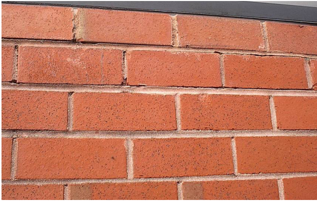
Photo 1 Mortar Joints in Need of Repointing
