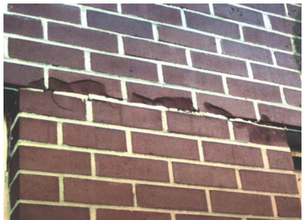
Photo 5 Spalling in Brickwork Without Horizontal Expansion Joint Due to Shortening of Structural Frame
