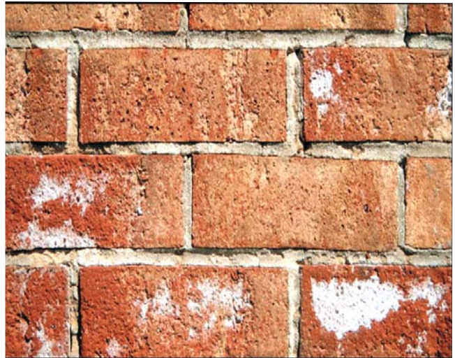
Photo 3 Efflorescence in Limited Areas
