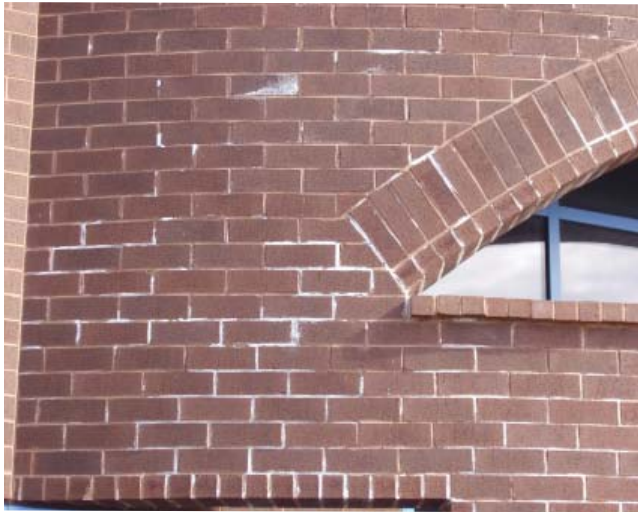
Photo 2 Efflorescence on Mortar Joints
