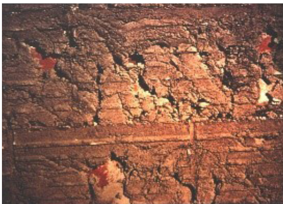
Photo 6 Poorly Filled Collar Joint
