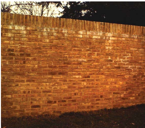
Photo 1 Efflorescence from Water Penetrating Wall Top
