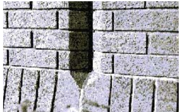
Photo 2 Accentuated Expansion Joint
