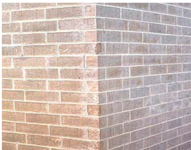
Photo 3 Spalling of Brick Masonry Wall with a Film-Forming Coating
