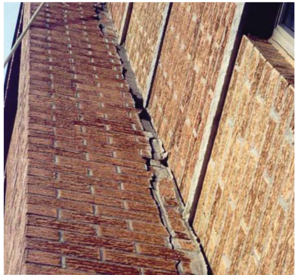
Photo 3 Crack at Offset Without Expansion Joint
