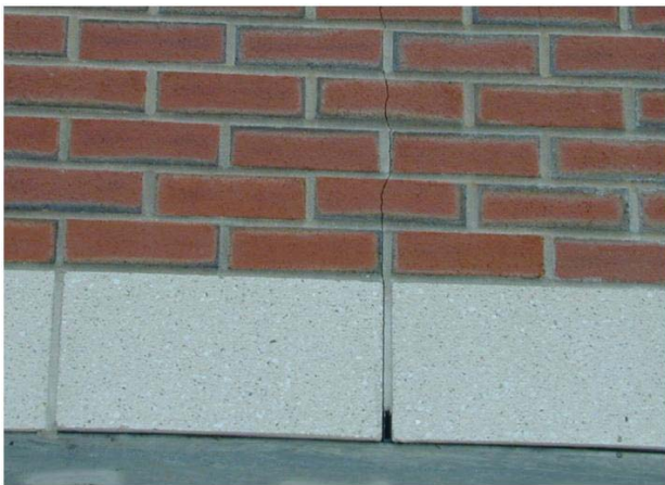
Photo 8 Crack Due to Deflection of Undersized Lintel
