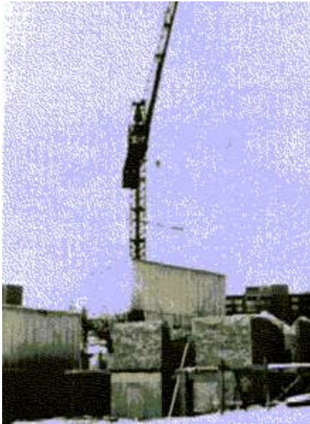
Temporary Enclosure at Jayhawker Towers, Lawrance, Kansas.
