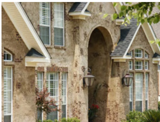
Photo 6 Mortar Wash Obscuring Areas of Brick
